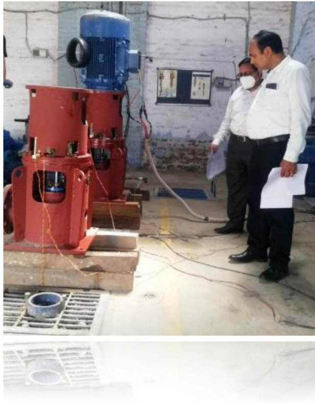
Inspection and testing of pumps done by Shri Vijay Kumar Assistant Engineer UPJN Aligarh
