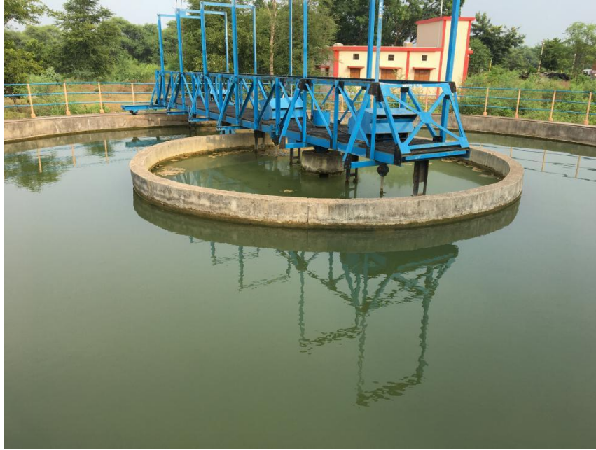
Supplied VT Pump in WTP Raipur P.H.E.D., Chhattisgarh
